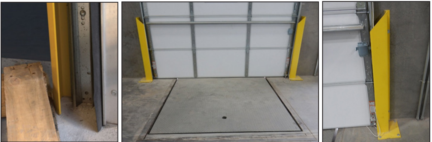
Example of a track door guards
