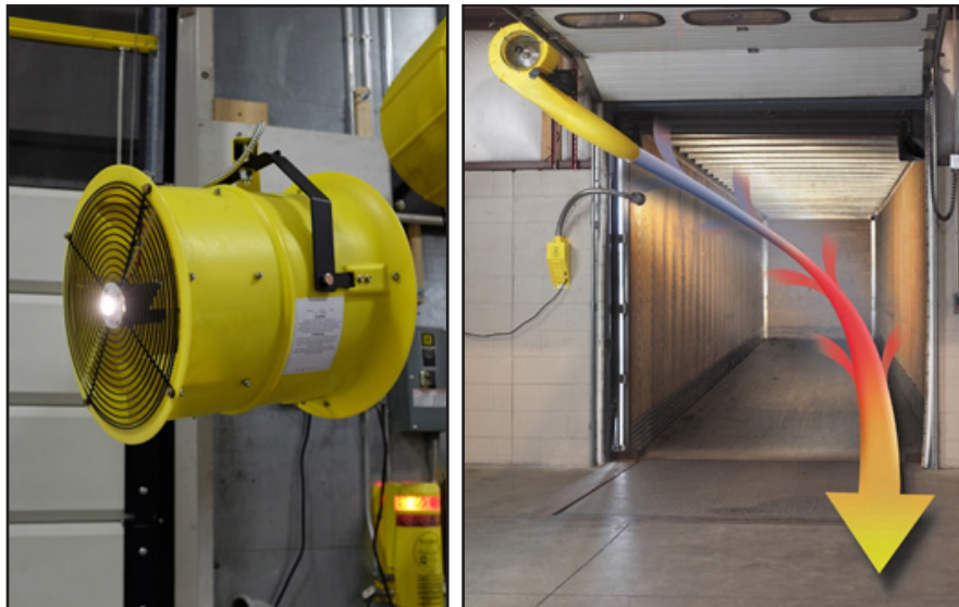
Examples of fans installed at loading docks
